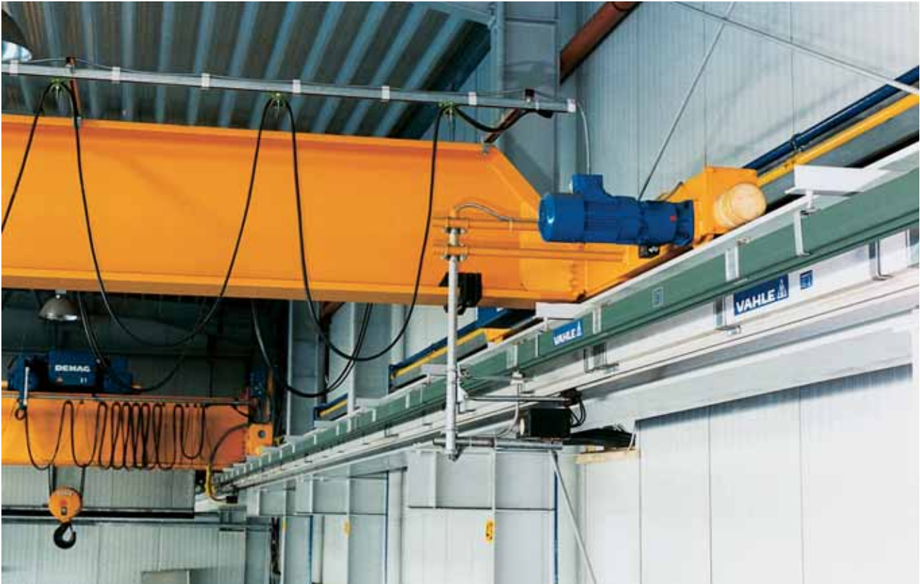
for downshop electrification.
